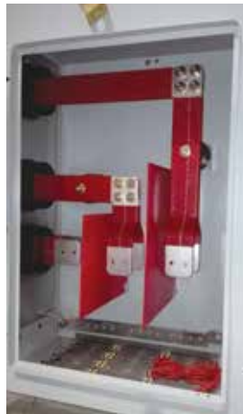
Figure 5.11: cable connection box
