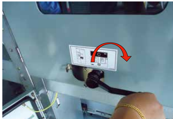
Figure 6.12: Rack in the breaker to work position
