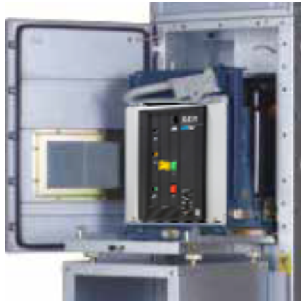
Figure 6.2: Transfer truck lock with switchgear
